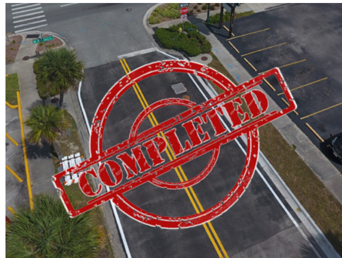
The baffle box located on Palmetto Street in front of Titusville Fire Department's headquarters and City Hall is now complete and traffic through the area has been restored.
