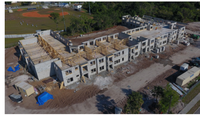
Construction continues on an 84-unit, 3-story apartment complex located at the southeast corner of Sycamore Street and DeLeon Avenue.
